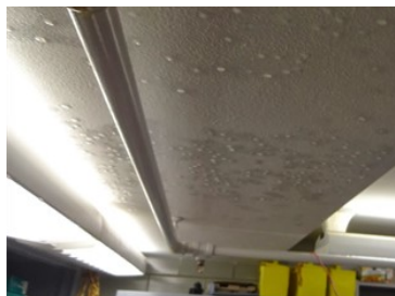
Figure 1: Water leaking through a lab ceiling from a flood above
